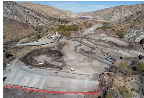
Crews building the grade control structure at the Littlerock Dam and Reservoir.
